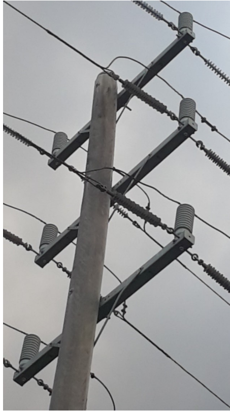
Figure 3.3: Overhead distribution power line insulators.
