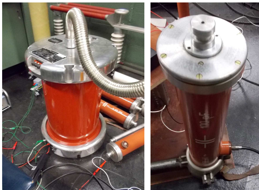
(a) Input transformer
