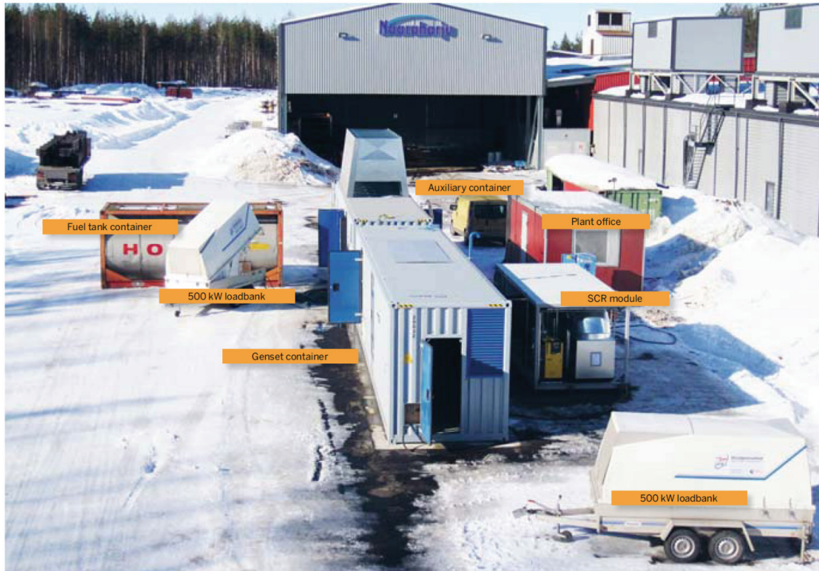
Figure 2.10 Pieksamaki research power plant (69)
