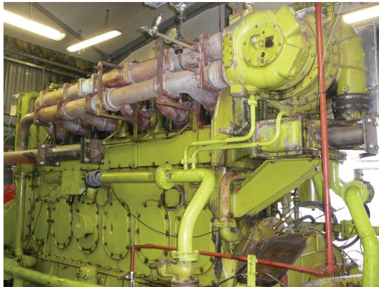
Figure 4.1 Ruston 6AR engine installed at John Pointon and Sons Ltd. premises at Cheddleton
