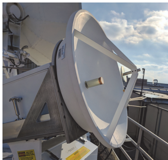
Figure 1. The hybrid beacon receiver and digital radiometer hardware under test at NASA Glenn Research Center in Cleveland, Ohio prior to deployment to the MDSCC in Spain
