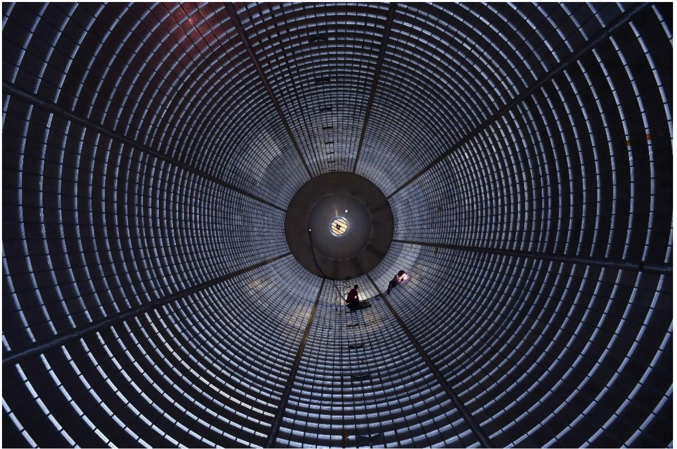
Fig. 2. Technicians inside an SLS core stage hydrogen tank plug fusion weld holes.
