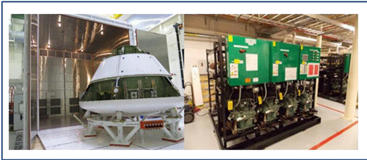
Figure-9- Thermal Cell in the Airlock and the Cell Support Equipment located in the O&C Basement
