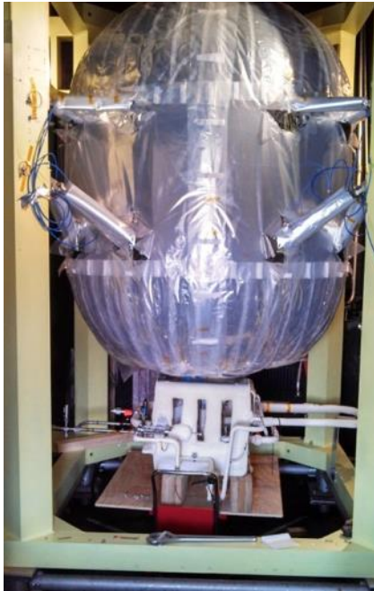
Figure 8: EDU tank as installed in TS 300.
