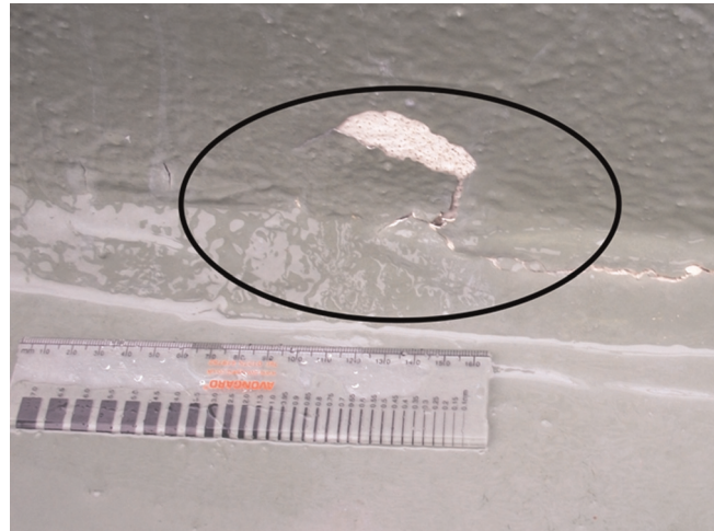
Figure 4. Cracking in the waterproof membrane between tower and foundation
