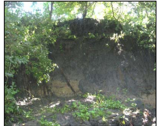
Photo A - Eroded Bank in Volunteer Creek
