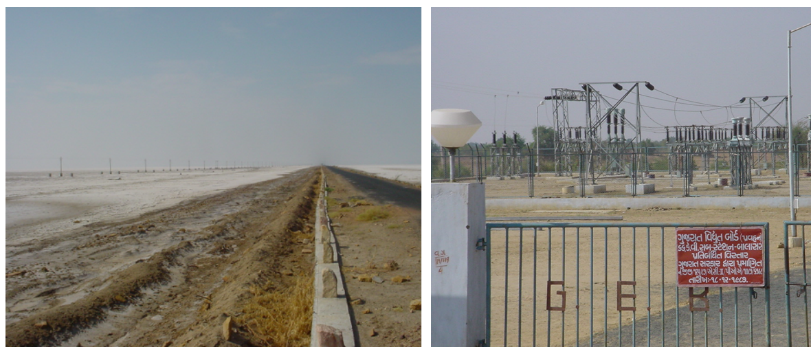
Figure 2.2: Transmission line across the Rann and GEB substation in Balasar
