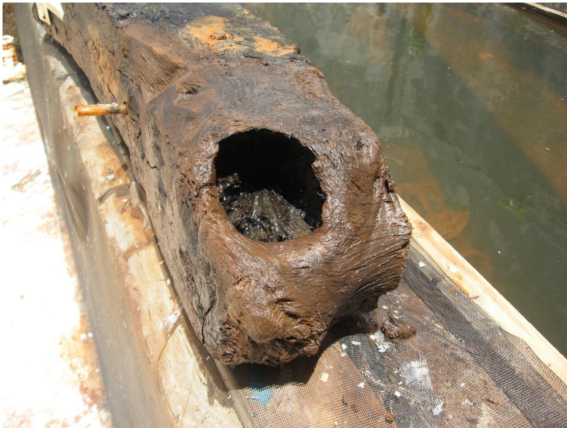
Figure 4.37: Inboard end of the deteriorated portside first futtock of third frame aft (FR 3 P1) showing knots and original branches.
