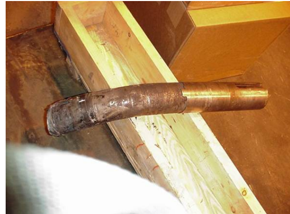
Figure 19. Bent Turbine Shaft Segment
