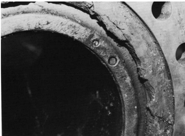
Figure 3. Sludge Lock up In Gear Coupling. (Calistrat)
