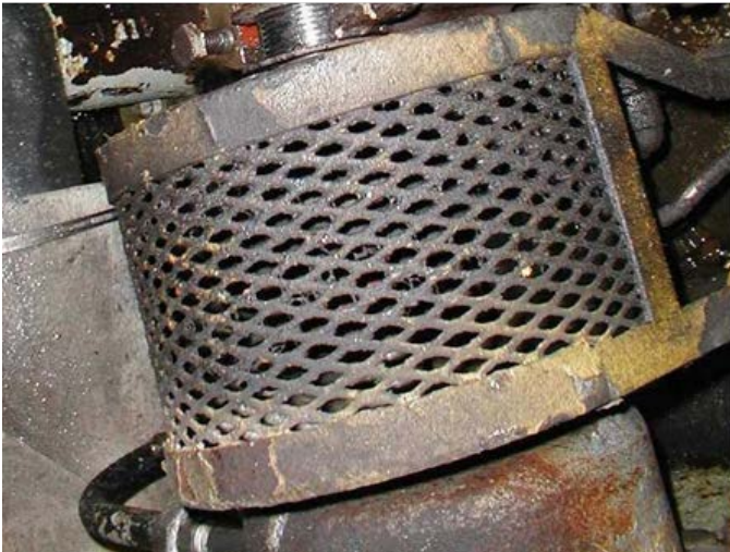
Figure 61. Grease displaced by water collects on guard made visible by an expanded metal guard. Solid guards hide leakage.
