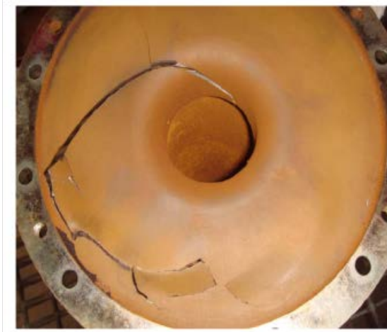
Figure 12. Excessive Torsional Oscillation Failure
