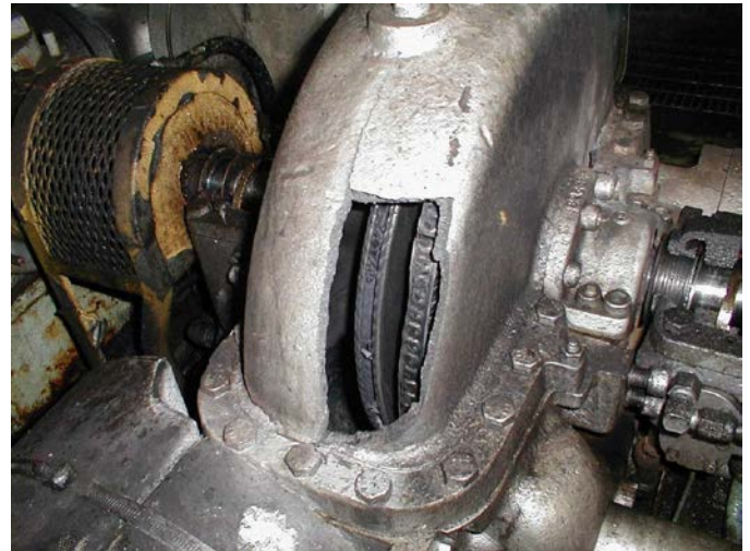
Figure 59. Turbine ran away after gear coupling failed
