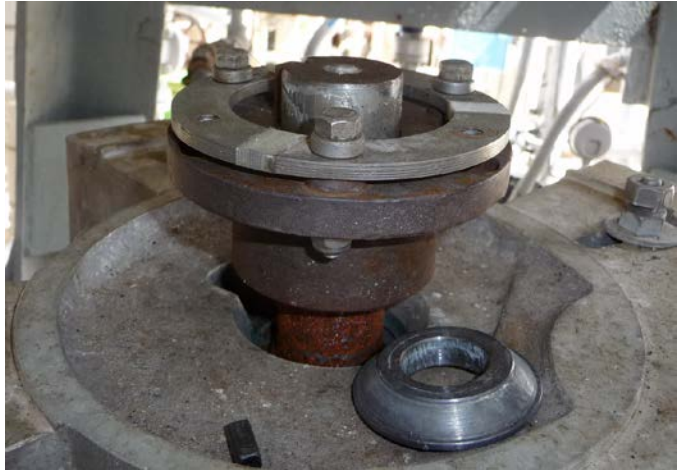
Figure 56. Hub was incorrectly modified to be a slip fit.
