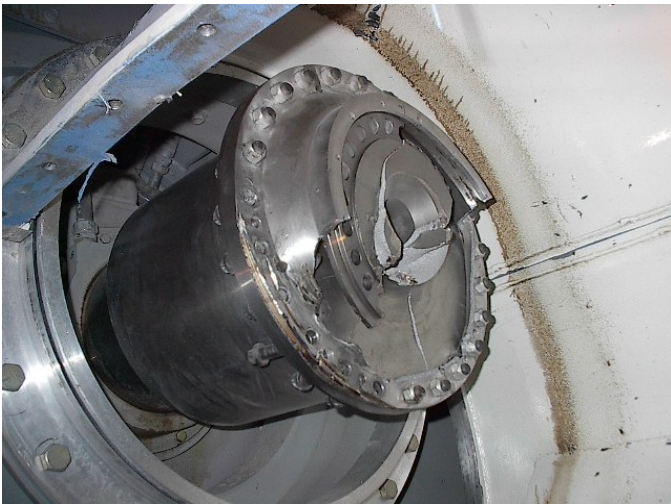
Figure 43. Broken Anti-Flail Guard
