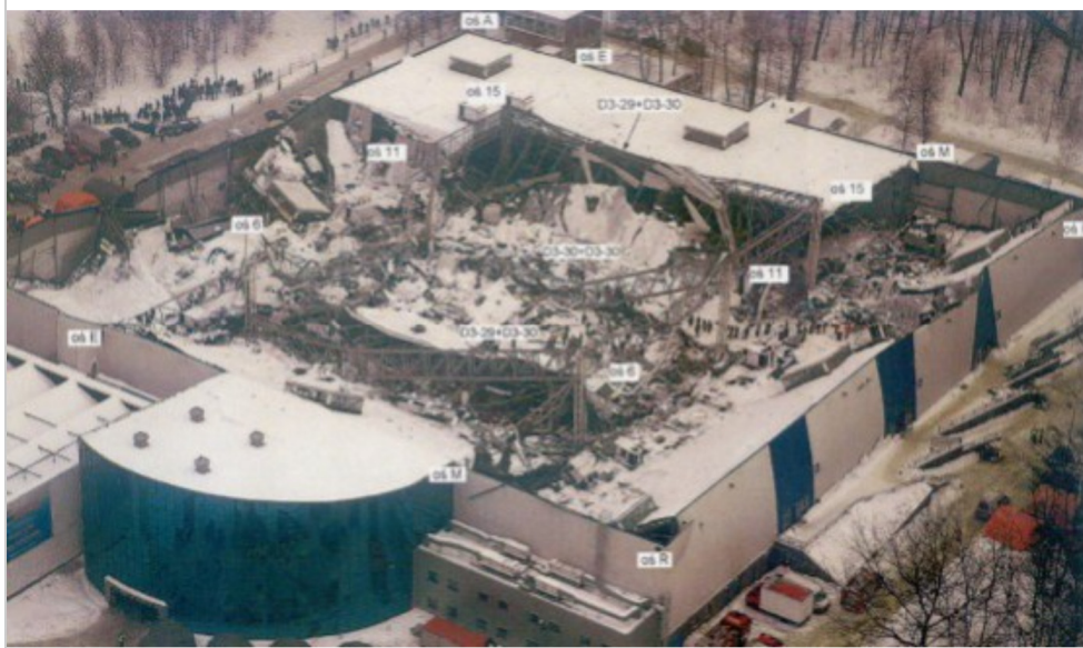
Fig. A – The collapse of the Katowice Exhibition Hall in 2006
