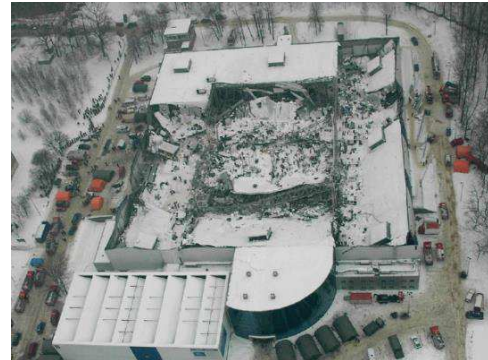
Figure 1. Roof collapse of Katowice Exhibition Hall
