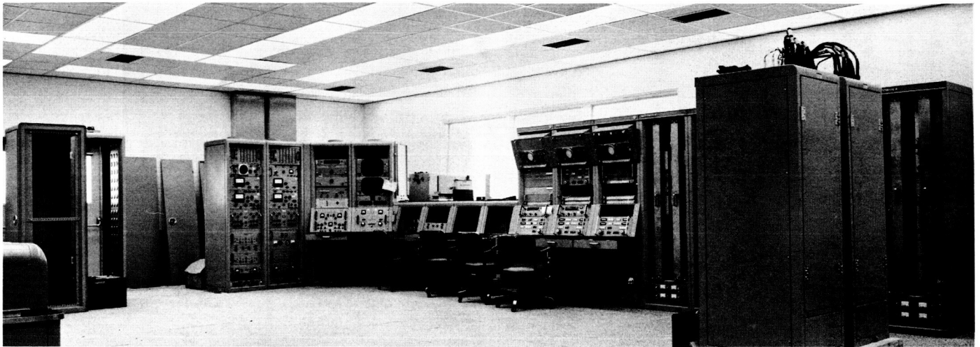
Fig. 2. Antenna servo and receiver installation
