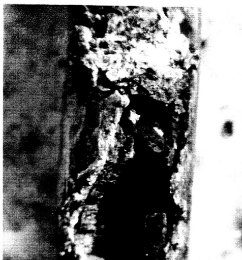
FRONT VIEW, CLOSE-UP OF RUPTURE NEAR END.
