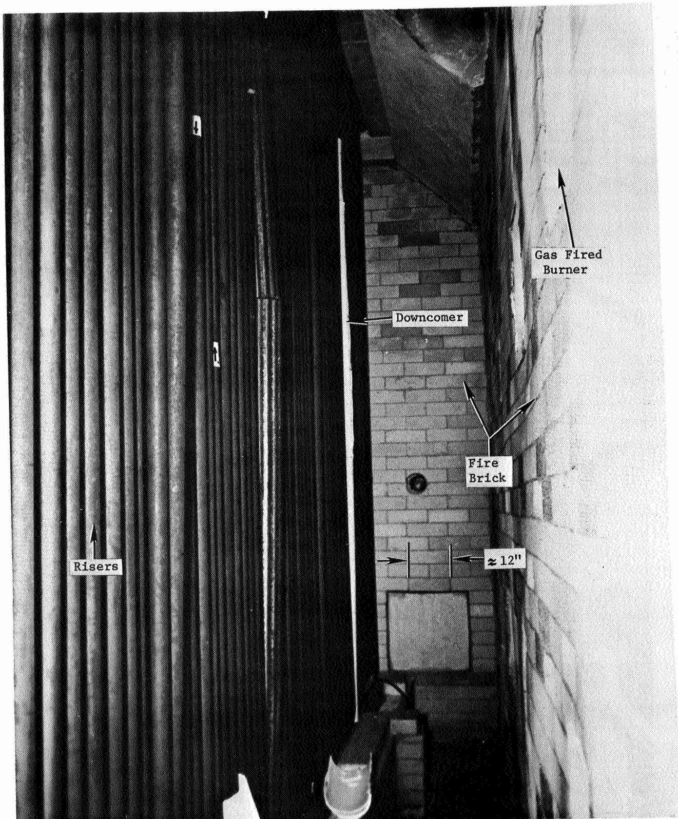
Figure 6. Boiler Tube Bundle.
