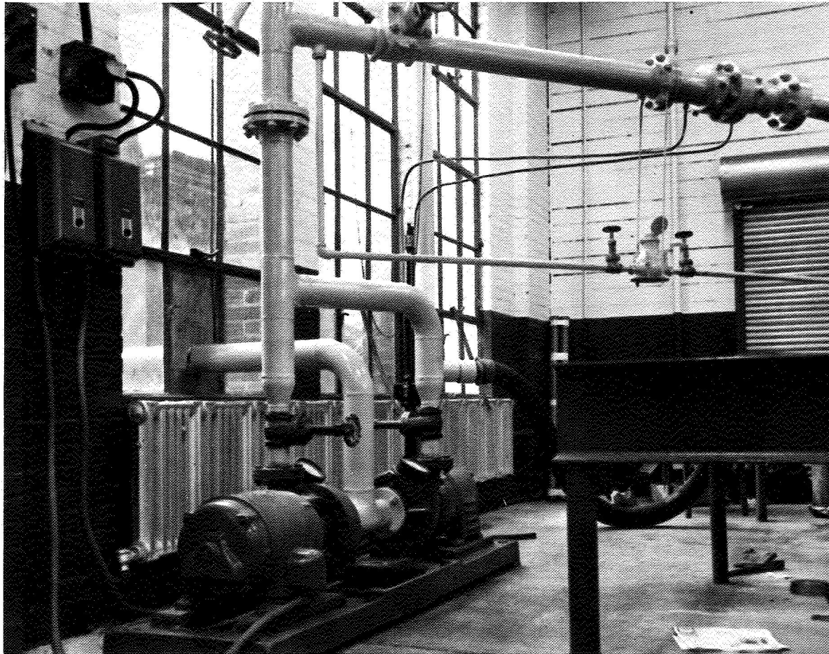
DATA PRODUCTION SYSTEM FOR WATER SHOWING PUMPS AND CONTROLS
