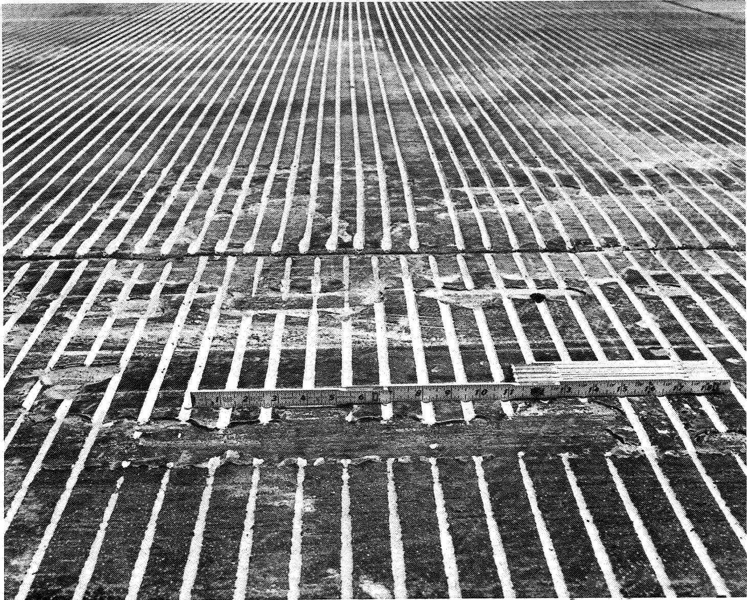
Figure 5.- Ungrooved areas left by peeling of paint and rubber deposits.
