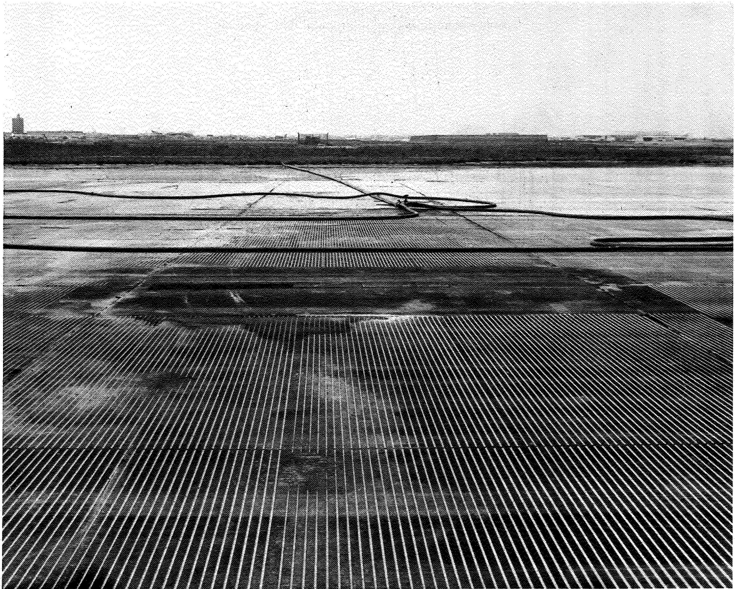
Figure 2.- Grooved runway with ungrooved slabs containing Elfaka light units.
