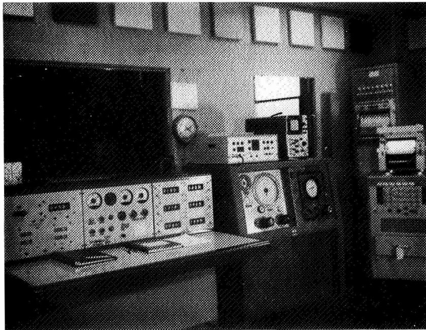
FIG. 4. Control Panel and Recorder
