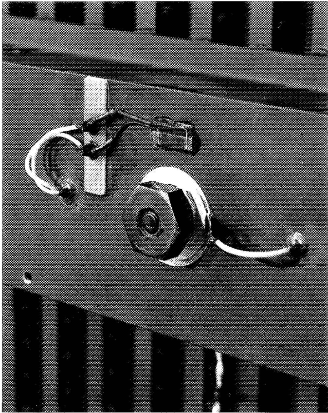
Fig. 7. Typical temperature transducer installation
