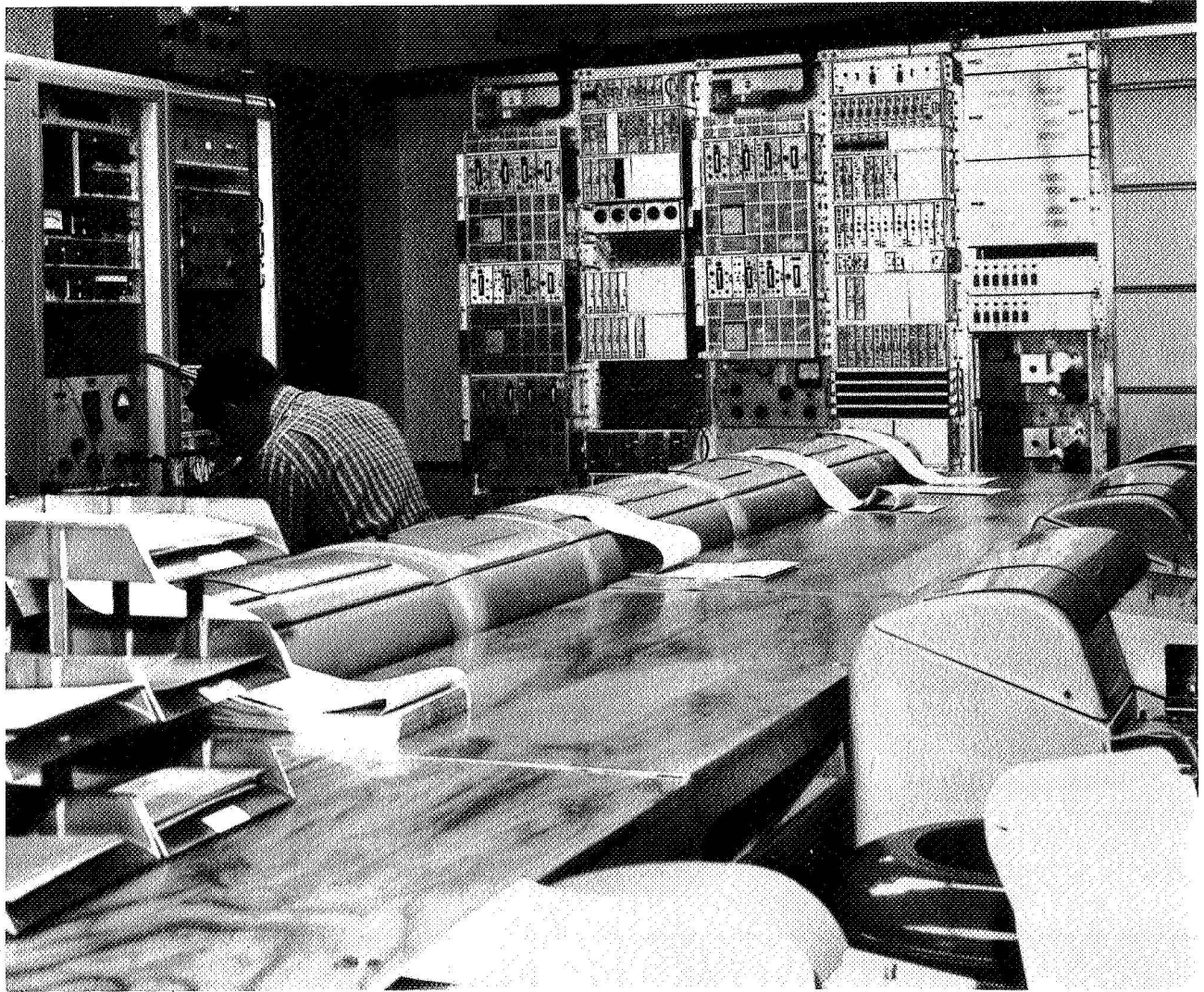
Fig. 14. Terminal equipment for MSFN intersite microwave system at Mars station
