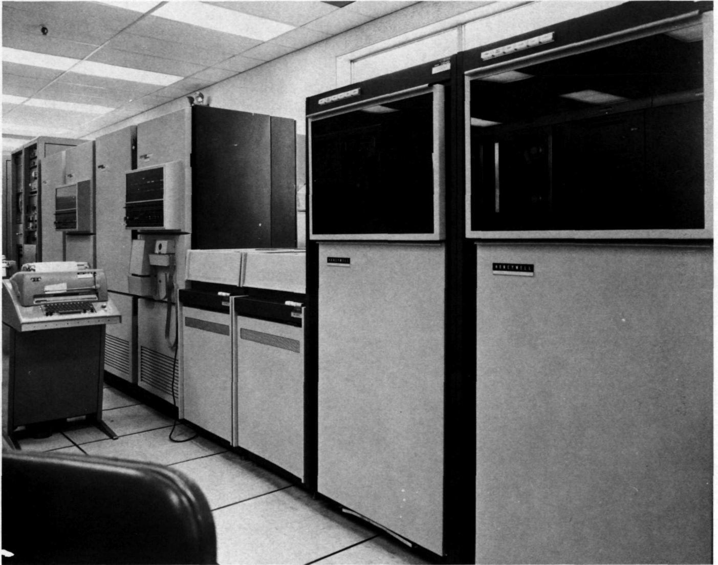
Fig. 4. DTS engineering model viewed from east end
