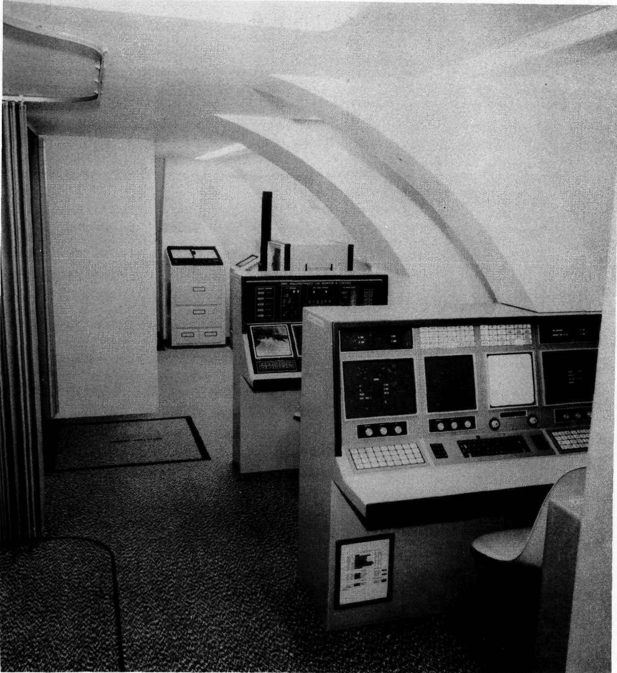
Figure 2-13. SM-1 Upper Deck, Control Center No. 1
