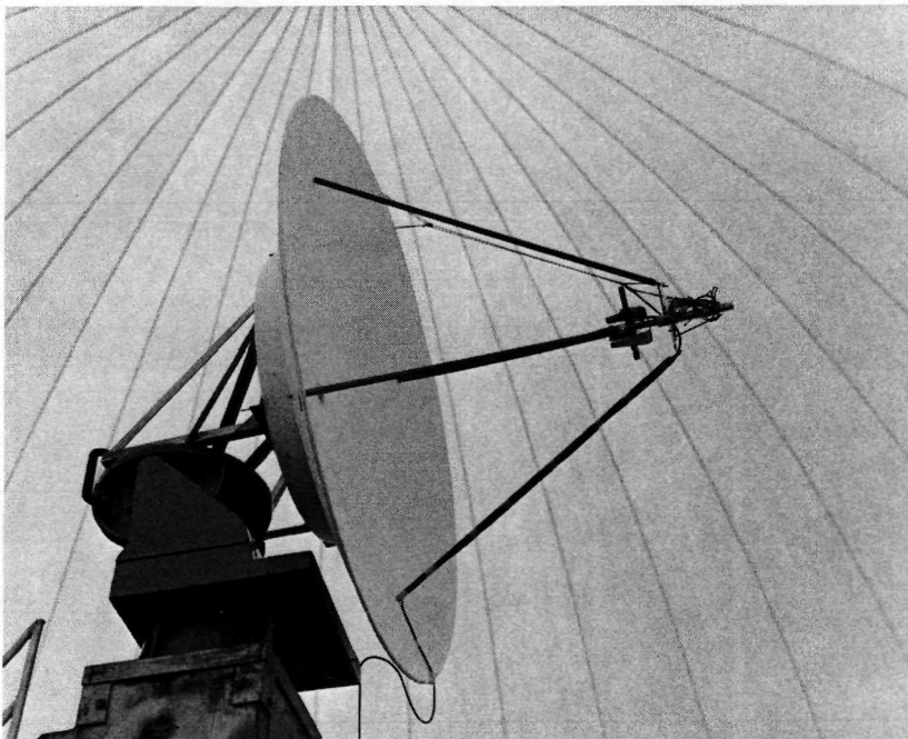
Fig. 117 Reflector with feeds on site at Santa Cruz Test Facility (View II)
