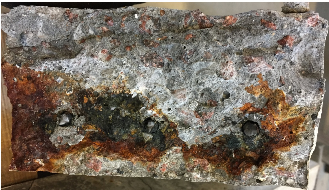
Figure 4.1. Image illustrating the formation of black rust around the reinforcement and the progressive change towards red rust as corrosion products propagated towards the concrete surface.
