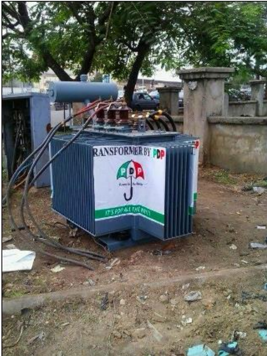
Figure 3.12: Electrical installations by PDP (People’s Democratic Party). Retrieved from: Facebook, 16 March 2015, posted by Abiyamo with the text, “PDP is using transformer to campaign in Cross River State, what do we call this?” URL:
