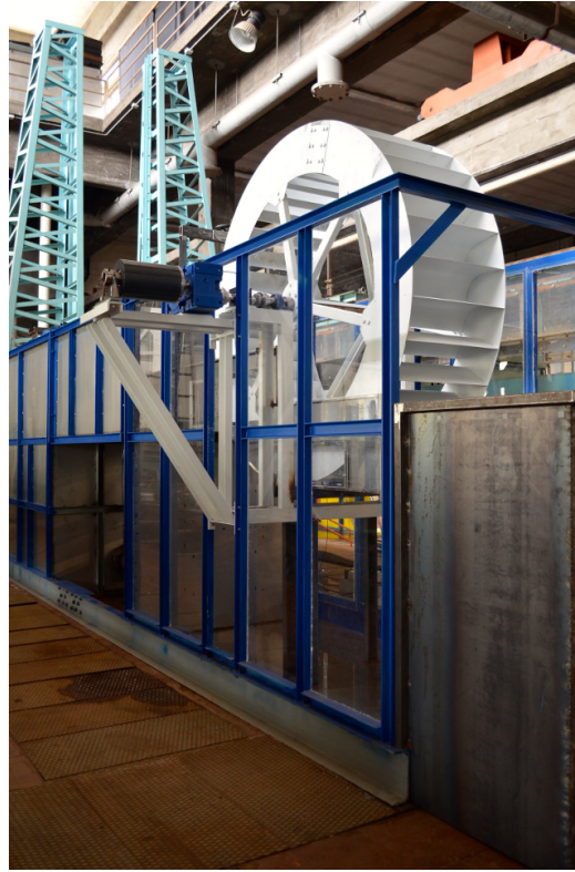
Fig. 3.4. The installed wheel with the gearbox (blue box) and generator (black cylinder).
