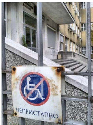
Figure 2. Inaccessible main entrance to the Faculty of Architecture in Skopje
