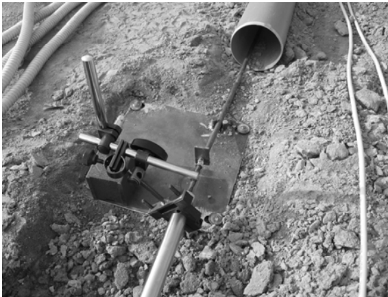
Fig. 8. View of the devices used for the measurement of the anchoring plate displacements.
