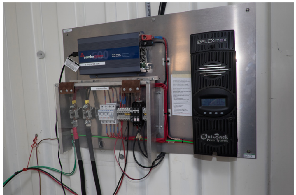
Fig 7. Electrical control plate inside of container.
