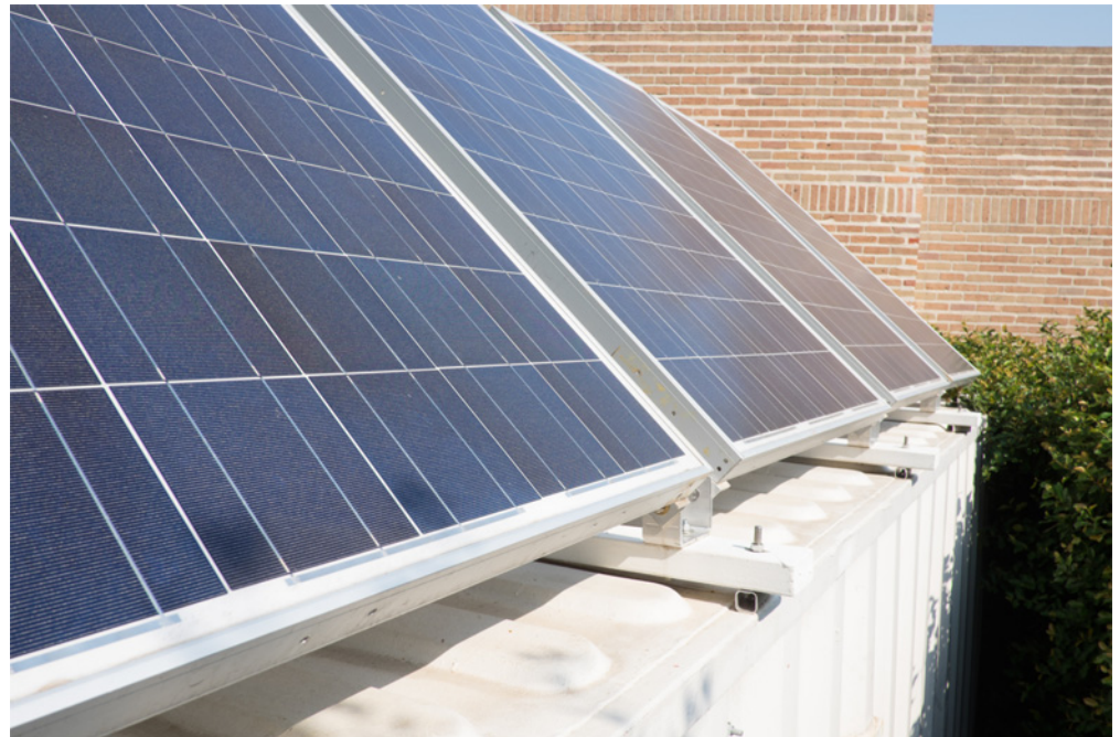
Fig 6. Solar PV panels mounted on container's roof.
