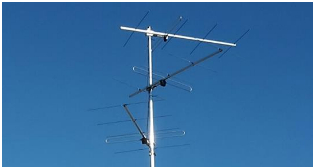
Figure 2.7: Yagi 5-element antennas rotated at an angle of 60 degrees relative to each other.
