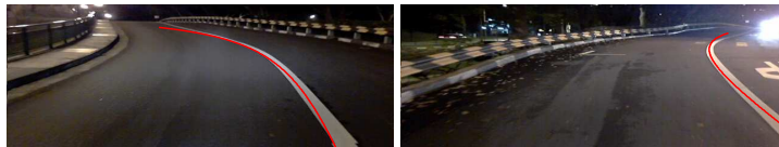
Figure 2.24: Inadequate model fitting examples (red lines) at non-flat road surface
