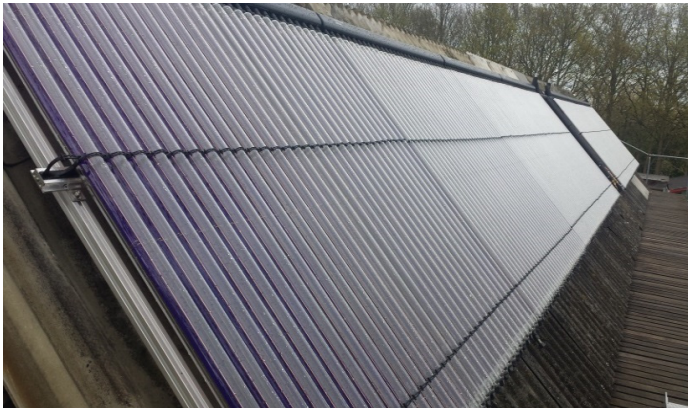
Fig. 2. The solar collector array consisting of seven Kingspan HP450 evacuated tubular solar collectors mounted on a south facing roof.
