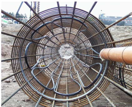
Fig. 2. Absorber pipes fitted to the reinforcement cage of a large-diameter bored energy pile
