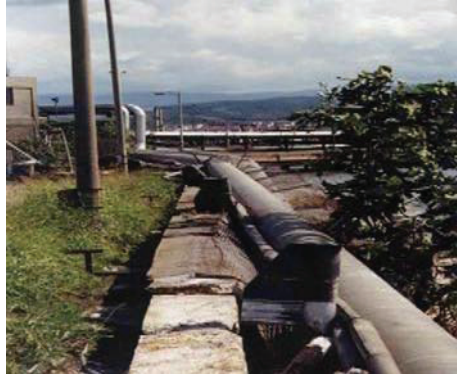
Figure 1: Damaged water pipeline in Tupras refinery
