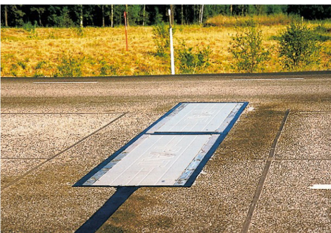
Fig. 5. HS-WIM bending plates installed in a road section.
