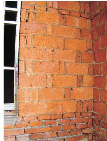
Figure 7 Poor quality of a masonry wall
