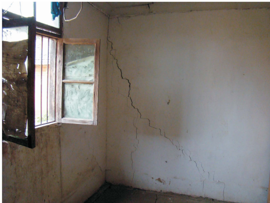
Figure 5 Wall junction vertical crack
