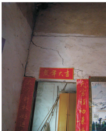
Figure 6 Wall tilt crack
