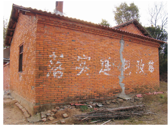
Figure 4 Wall vertical crack
