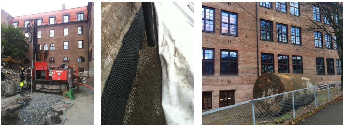
Fig. 4. (a) Digging for the ground source heat. (b) Combined digging for collector pipes, exterior insulation and drainage. (c) The oil tank on the way to destruction. Photos: G. Andersen, September 2012.
