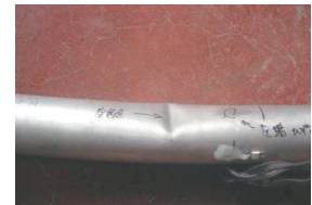
Fig.4. Failure of hollow single-wall pipe.
