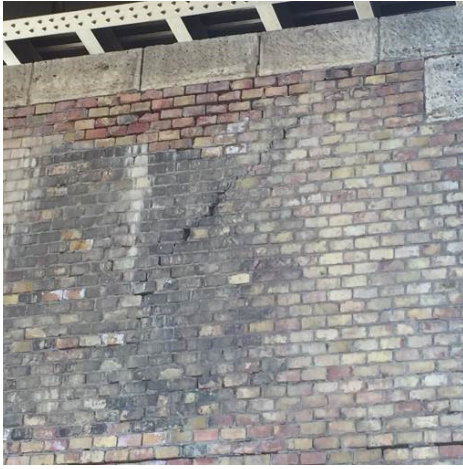
Fig. 8. River pier, cracks, mortar rinsing
