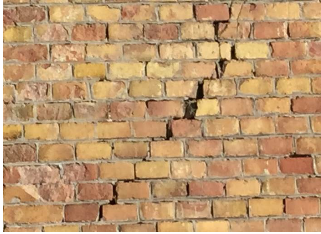
Fig. 9. River pier, aslope crack, crushing and cracking of brick elements
