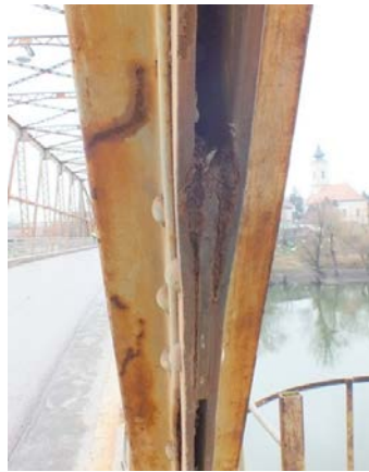
Fig. 3. Delamination and spalling of steel due to corrosion, swelling and expansion of steel profiles
