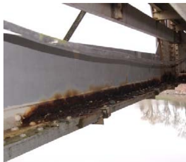
Fig. 6. Appearance of transverse girder, corrosion in lower part of vertical steel sheet
