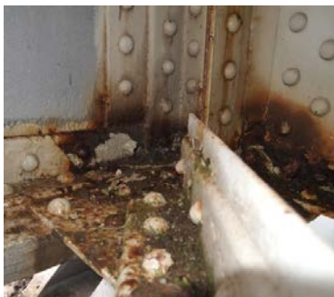
Fig. 5. Corrosion at the junction of main longitudinal and main transverse girder, reduction of cross section of steel profiles
