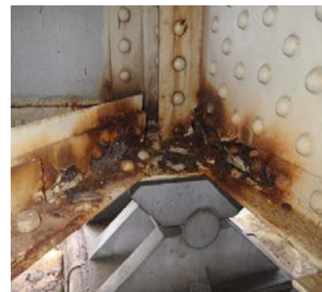
Fig. 7. Appearance of the supporting zone, corrosion
