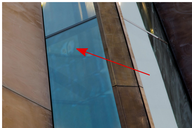
Figure 2 Visible anisotropies at a façade glazing; single spots.
