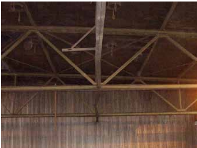
Fig. 2. Deformation of chords of the longitudinal bracing at the gable wall [3]. The horizontal deviation measures 170mm, which makes about 1/50 of the span. The load-bearing capacity of the member fell under 20% of its original capacity. The deformation of the bracing indicates that it could be loaded by horizontal actions from the gable wall.
