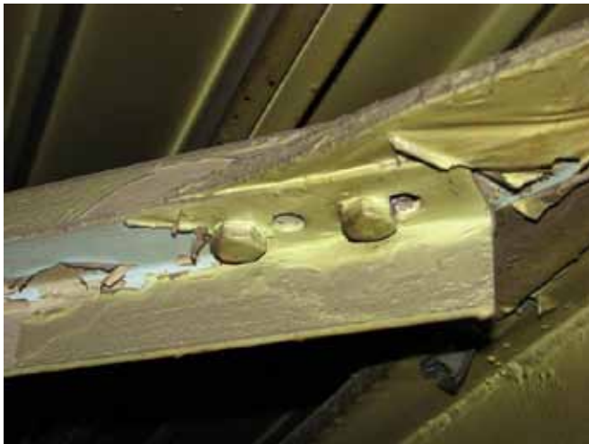
Fig. 4. Wrong drilling of the bolt connection of a cross roof bracing diagonal as a consequence of inaccurate assembly of the structure [4]. The load-bearing capacity of this connection reaches only about 60% of the designed connection capacity.
