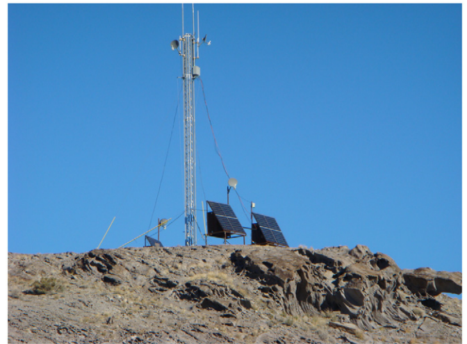
Fig. 5. The Smelter Knolls communication tower, one of three in the array. There are three stands each with four solar panels. Those stands contain batteries, data acquisition PC and network instruments for long distance link.
