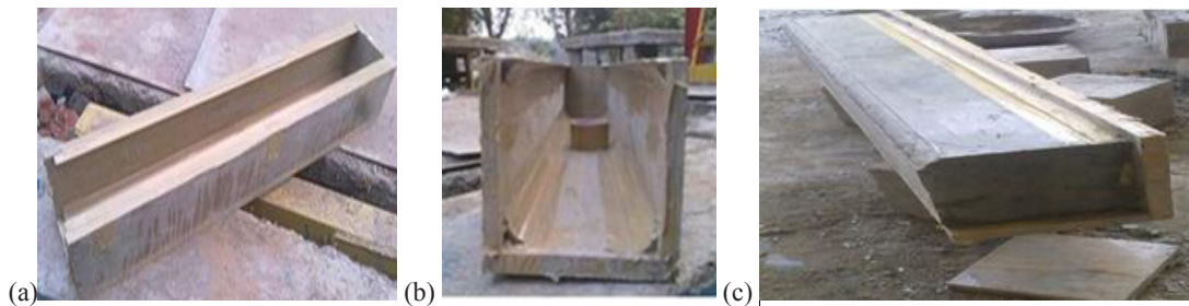
Fig. 3 (a) Formwork for column with corner radius 20 mm, (b) Completed formwork with corner radius patty and (c) Formwork with cast specimen.
