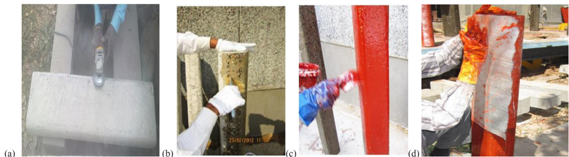
Fig. 4 (a) Grinding of RC column, (b) Application of Primer, (c) Application of saturant and (d) Application of GFRP sheet
