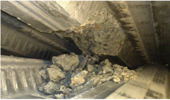
Fig. 11. Cone failure surface indicative of pull-out failure in left half-span of 10 m specimen.
