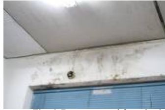
Fig. 6. Dampness and fungalstain
