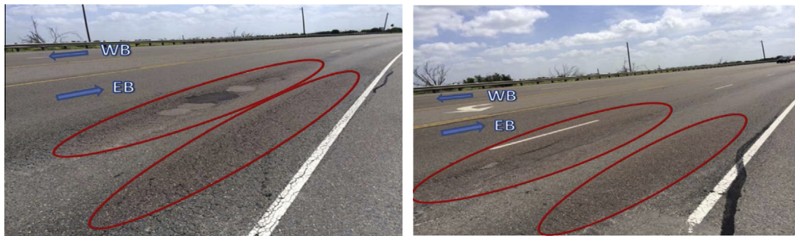
Fig. 13. Pavement surface condition of FM 1016 in summer 2015.
