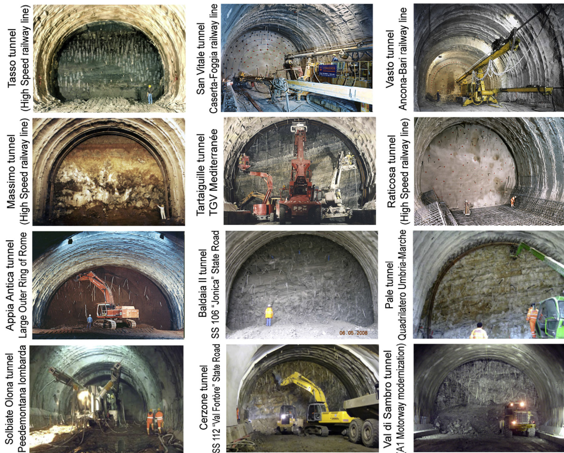
Fig. 2. Photographs showing the face of a few selected tunnels excavated full-face by using the “heavy method” (Lunardi and Barla, 2014).
