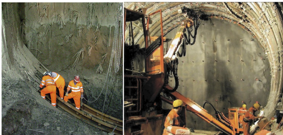
Fig. 6. Full-face excavation and construction method: face reinforcement and ring closure: “heavy method” (left) and “light method” (right).
