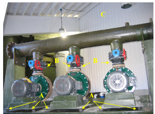
Fig. 8. A custom pump stand fabricated by Marine Biotech Inc. (Beverly, MA) installed at the USDA ARS, NCWMAC (Franklin, ME) illustrates (A) resilient pump mounts to reduce transmission of motor vibration noise, (B) rubber vibration isolation couplings on both the pump inlet & outlet piping, and (C) locating the water treatment pumps and equipment in a room separate from the fish culture tanks.
