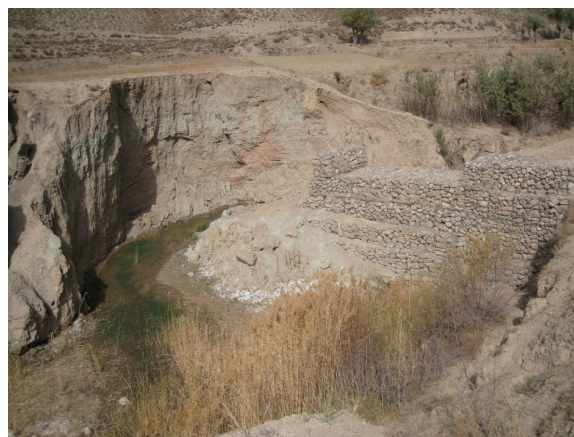
Fig. 5. Stone gabion after head cut.
